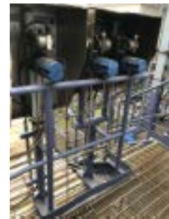
FIG 3 Three Yokogawa transmitters installation.
