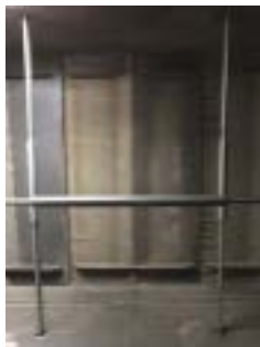
FIG 1 VERIS Verabars® V510-15 sensors in front of duct louvers.
