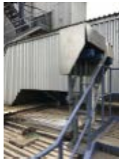
FIG 2 Transmitter installation showing impulse lines and isolation valves coming off the VERIS Verabar® sensors.
